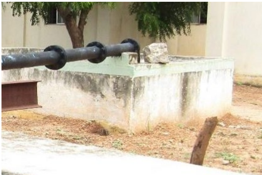
Figure 2.4: Grit collection pit
