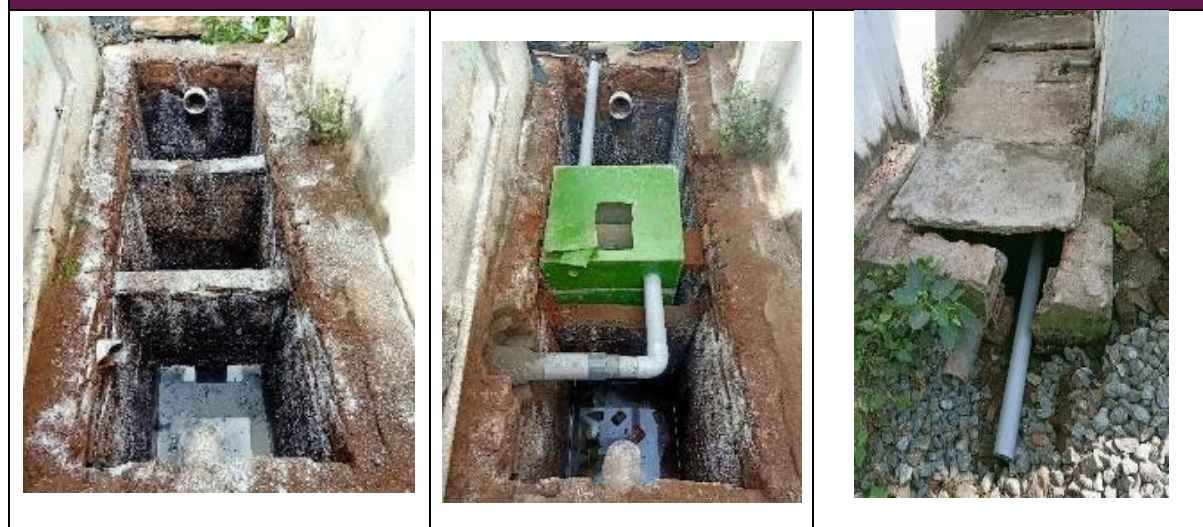
Figure A5.5:DRDO Biodigester (FRP) post installation
