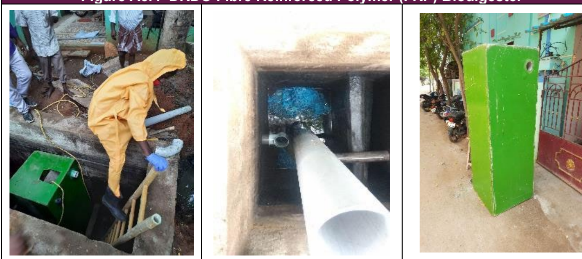
Figure A5.4 DRDO Fibre Reinforced Polymer (FRP) Biodigester
