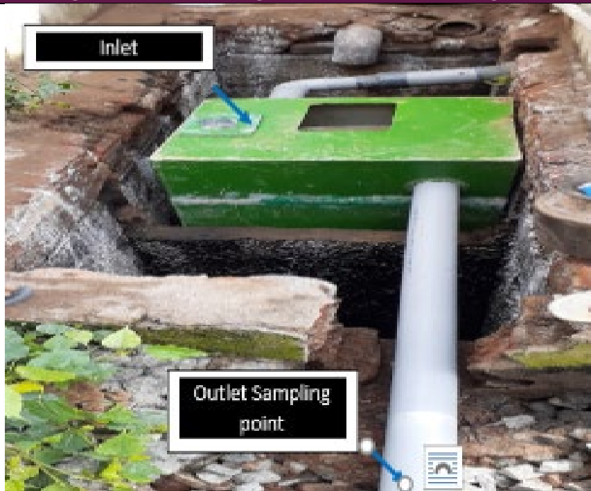
Figure A2.7: Sampling Points for DRDO Biodigester
