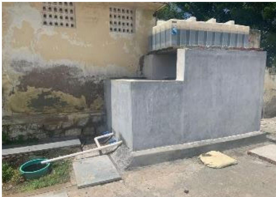
Figure 3.12: Current upgraded EBR at Thulasinganagar
