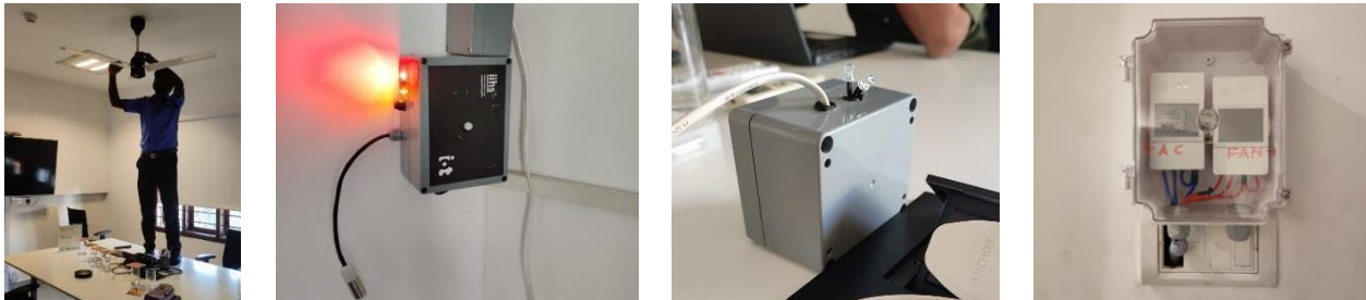
Figure 2. Images of the hardware installed in each room (a) BLDC ceiling fan, (b) IEQ box, (c) IR blaster, (d) energy meters
