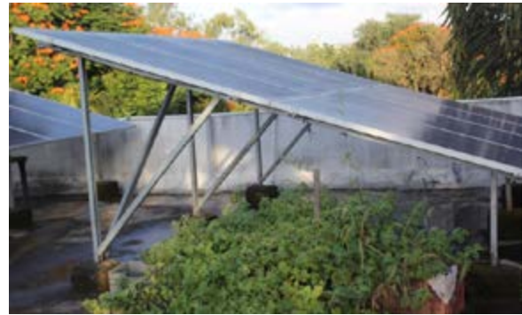
Figure 8.1: Roofs as multifunctional spaces—solar panels, rainwater harvesting, and vegetables all find place in PMC's Ghole Road office rooftop Source: Maitreyi Koduganti, September 2021
