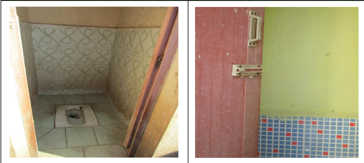
Figure 3.6: Cubicles with Missing Doors and Broken Latches
